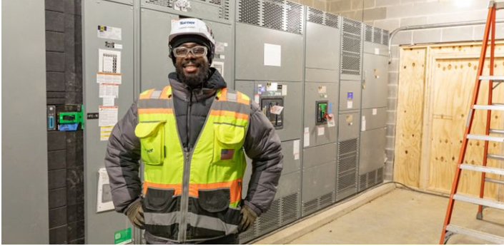
Electrical Switchgear Power Supply
