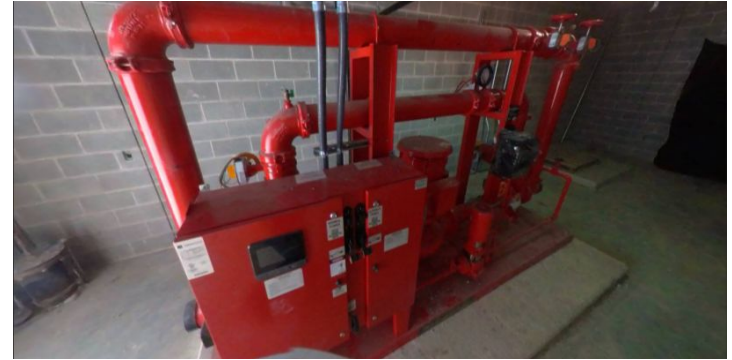
Sprinkler Pump Room
